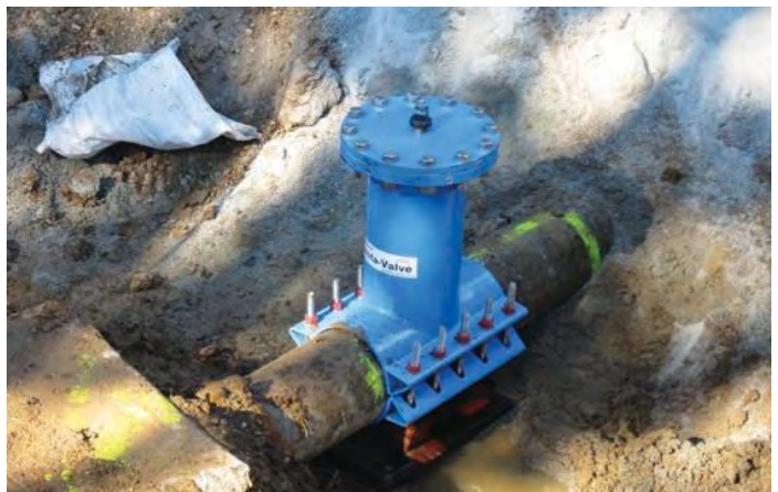
Insta Valve Kilcoy QLD
