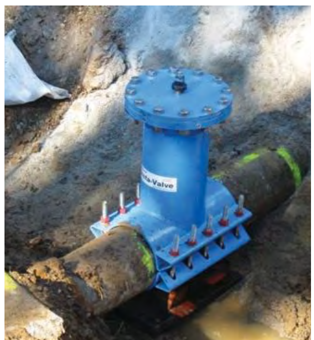
Insta Valve Kilcoy QLD
